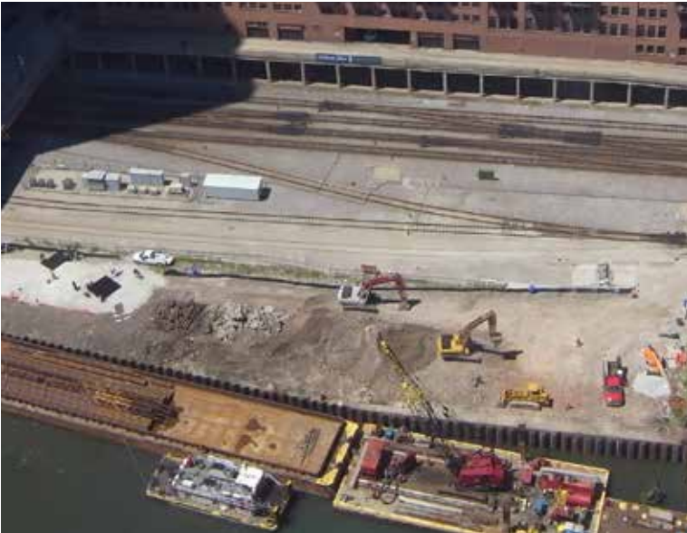
The 150 North Riverside site, shown during excavation, is hemmed in by a combination of barriers, including the city's set-back zoning requirements along the Chicago River and a seven-line Amtrak right-of-way. Photo: Goettsch Partners
