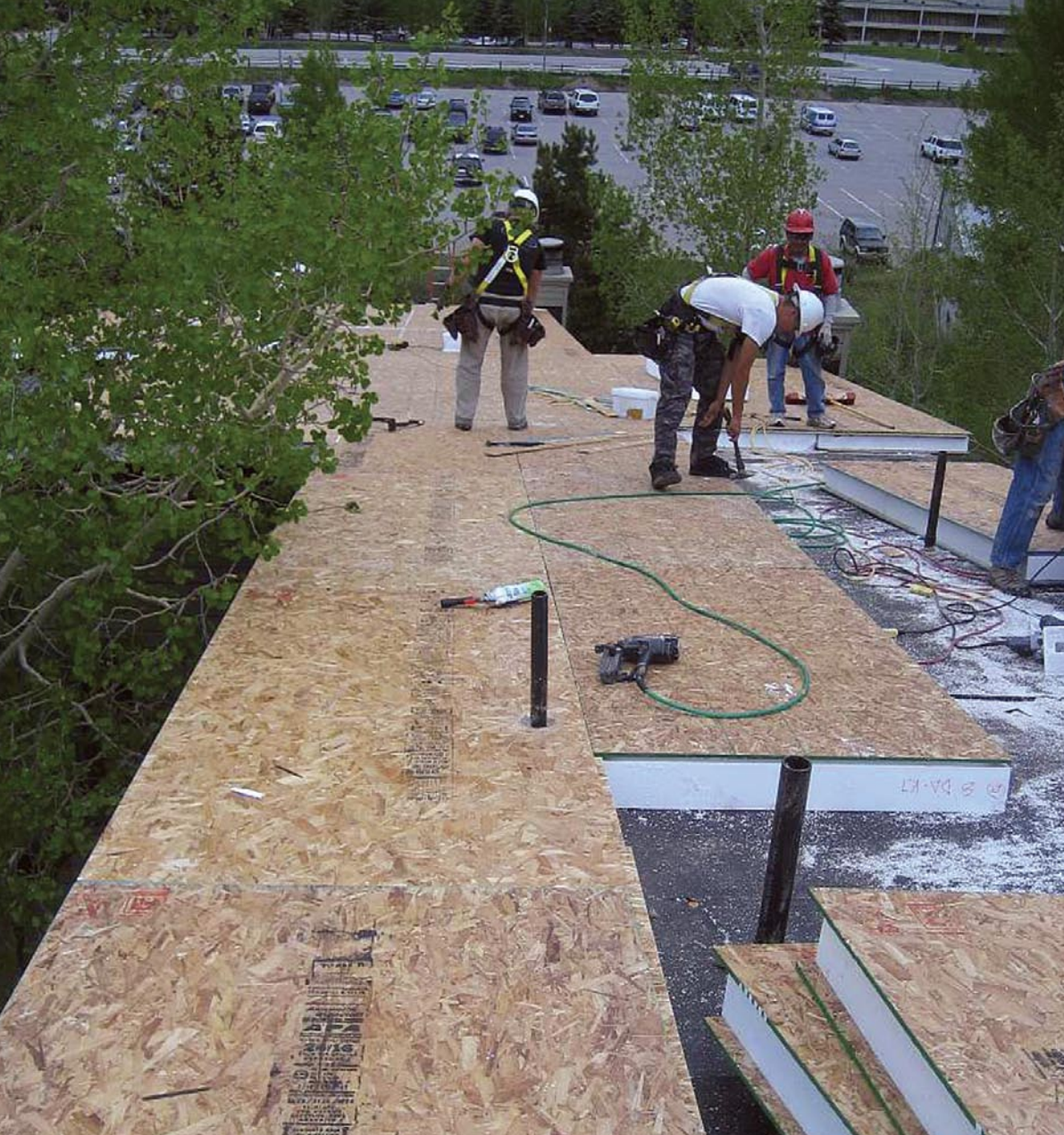
R-Control Structural Insulated Panels were installed along the perimeter of the building while Foam-Control Nailbase Panels covered the center of the roof.
